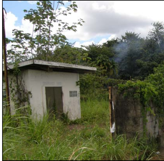
Photo 3.8: Santa Rosa Springs Lift Station
