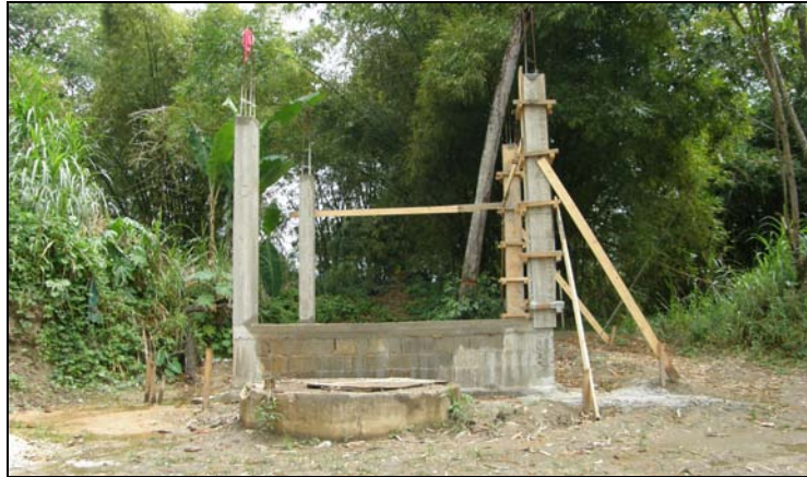
Photograph 3.6: Dundee Lift Station
